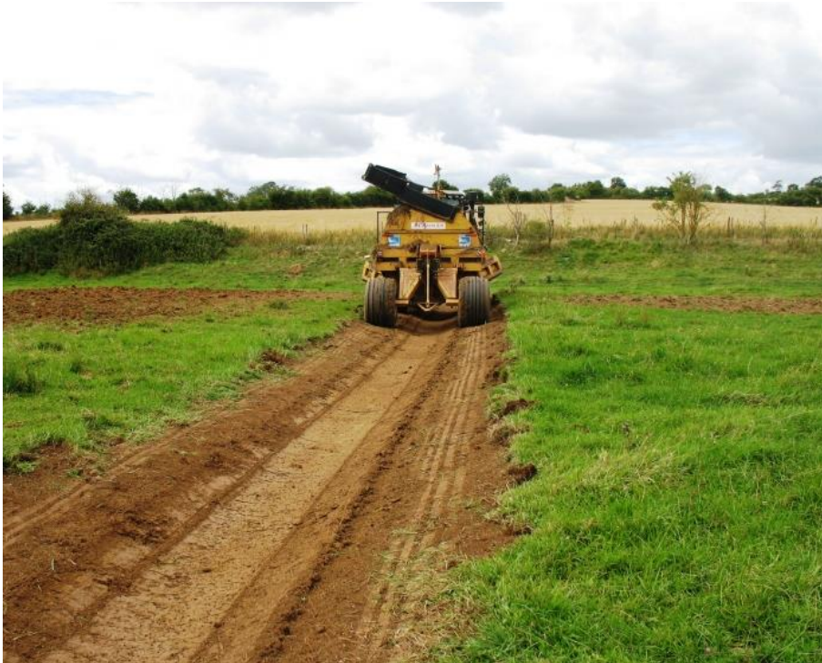
Figure 7: RSPB Rotary Drainer excavating a foot drain – the depth and width of the feature and spoil spreading can be adapted for use in the restoration of grips and furrows.
